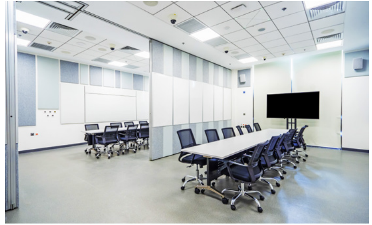
Meeting spaces such as this debriefing room enable students and staff to review exercises and training scenarios captured with an Extron SMP 351 streaming media processor.
