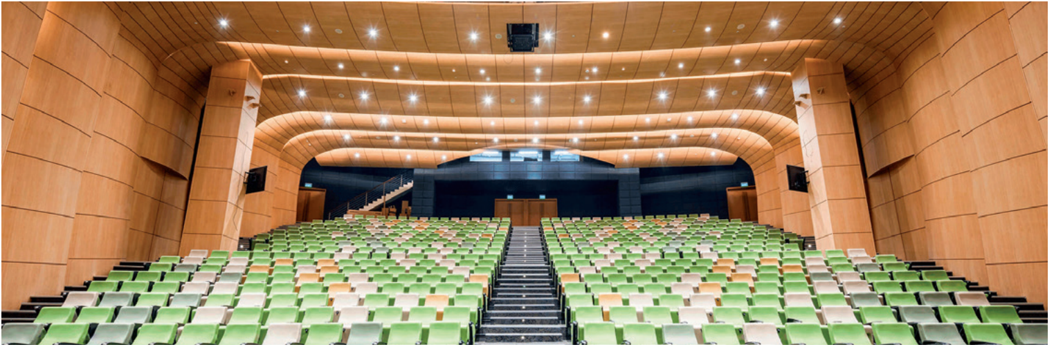
Auditorium has ceiling-mounted projector for the on-stage screen plus 55" flat panel displays in the audience seating area.
