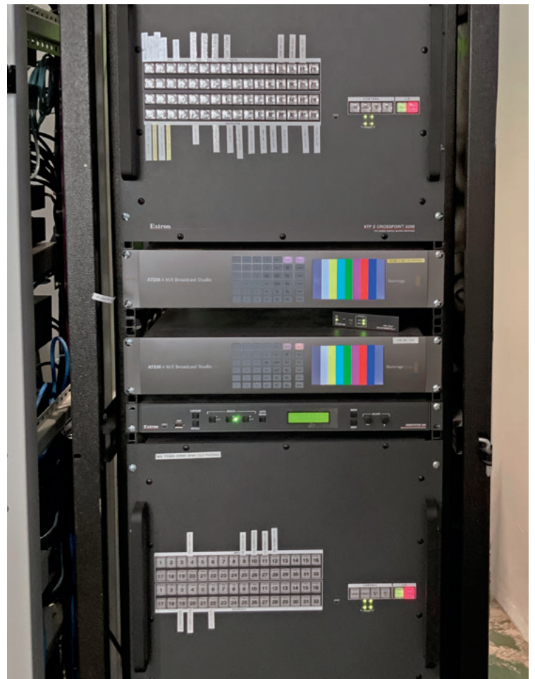
Auditorium AV equipment rack housing two XTP II CrossPoint 3200 Matrix Switchers.
