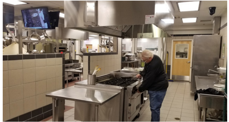
The culinary classroom includes six full commercial kitchens, and the instructor is a professional chef. A NAV Pro AVoIP system enables signal distribution to the various displays.
