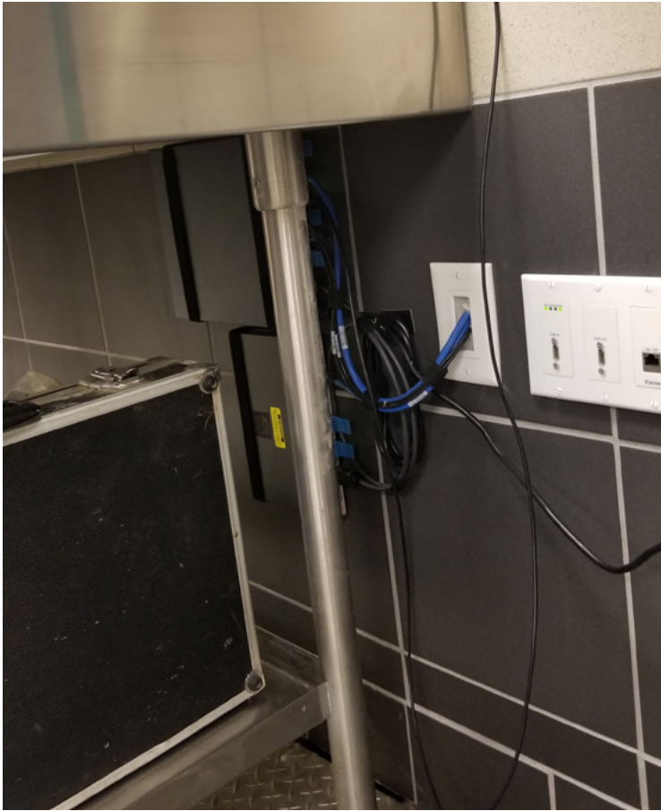
Located on a shelf beneath one of the preparation tables are the chef's PC and an Extron MediaPort 200, which converts the PC's USB signals to HDMI and then scales the video to enhance the content for the students attending from home.
