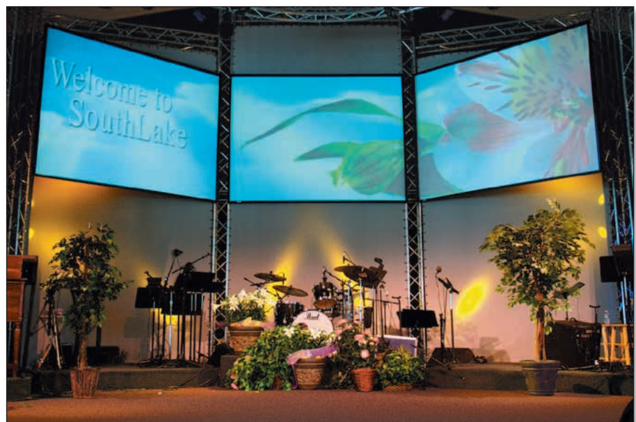
SouthLake's innovative AV system is integral to the sanctuary's main stage .
