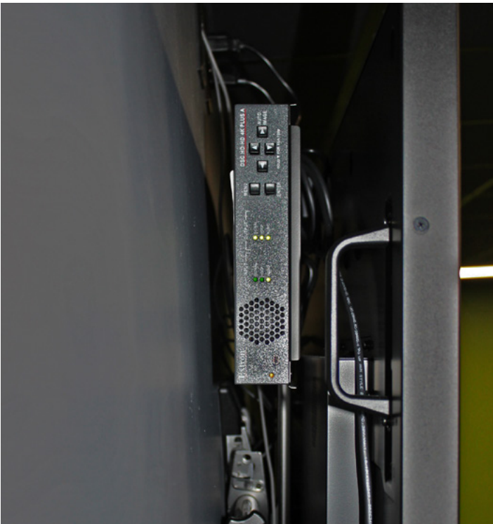
The DSC HD-HD 4K PLUS A mounted behind each wall display scales the 2560x1440 signal from the gaming PC to the display's native resolution. The scaler for the center display also de-embeds audio to support the sound system.
