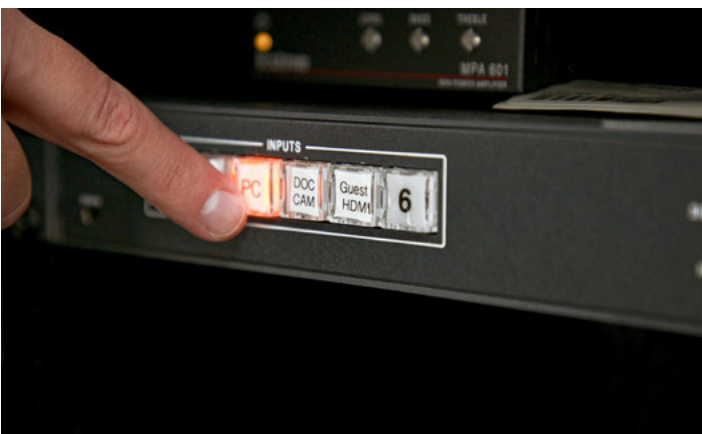
The switcher's clearly labeled buttons that light when pressed make AV source selection easy. Buttons 1 and 6 are spare inputs that allow future expansion.
