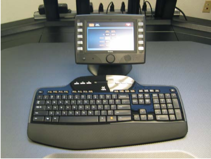
Extron TLP 700TV TouchLink Touchpanel controlling a SCADA workstation
