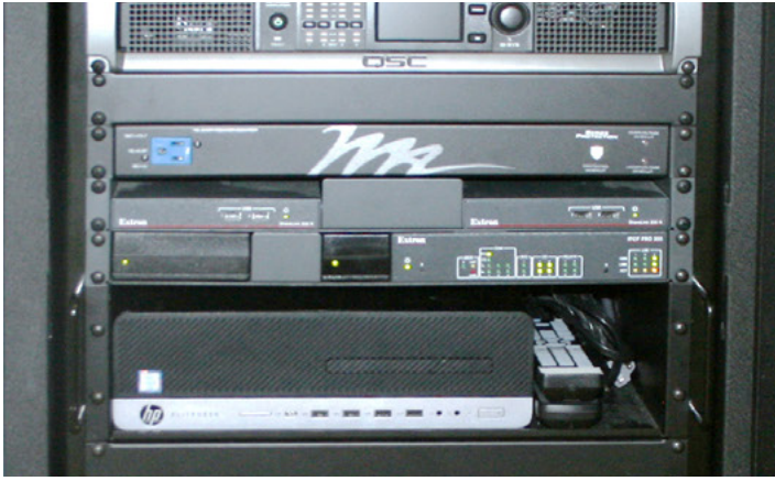
To switch and distribute AV signals throughout the HRM Culinary Arts facility, an Extron XTP II CrossPoint 3200 matrix switcher is rack-mounted within the central equipment room.
