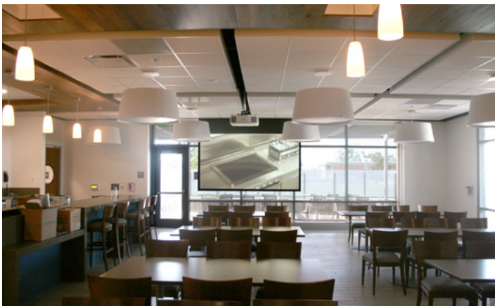
XTP CP 4i 3G-SDI boards installed in the modular matrix switcher accept live feeds from the PTZ camera system, enabling lecture capture for distribution over the twisted pair cable infrastructure and archival purposes.
