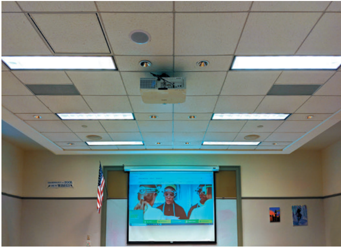
Three-year rollout of PlenumVault AV systems and VoiceLift Pro voice reinforcement microphone systems equips every classroom by Summer 2020. In this image the PlenumVault system is hidden in ceiling just to the left of the round speaker grille while the projector is flanked by two FlatField speakers.
