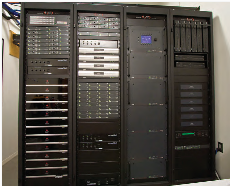
All signals are routed to the central switching room, which houses the twisted pair transmitters and receivers, Matrix 6400 switcher, and the codec farm.
