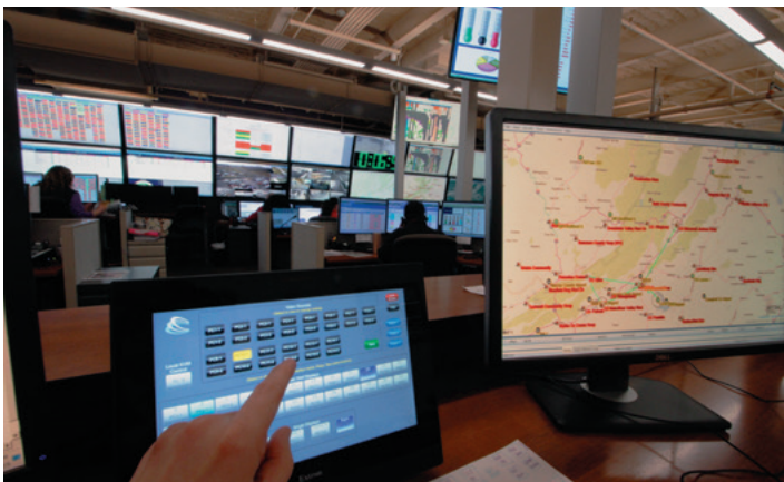
The CTaC manager uses the Extron TLP Pro 1220TG Tabletop TouchLink Pro Touchpanel at their desk to easily control the XTP system and select the content for each of the 28 wall-mounted displays.
