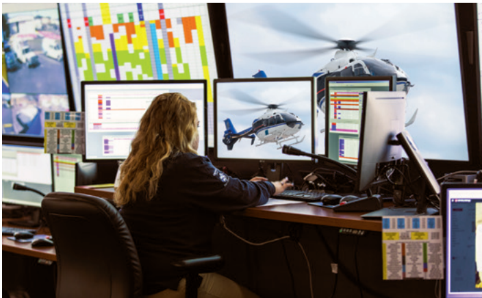
The XTP system enables source signals to be sent to any combination of the 28 flat panel displays mounted across one long wall in the rectangular room. The XTP II CrossPoint 6400 remotely powers the XTP receivers over the CATx cable.
