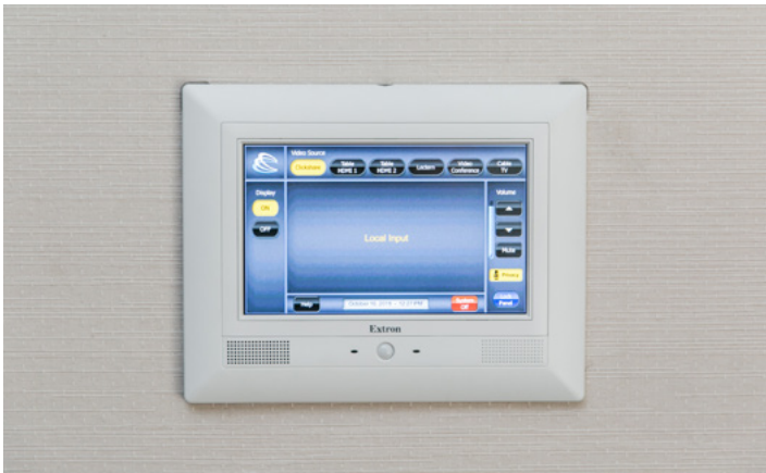
The Extron DTP CrossPoint 84 4K IPCP MA 70 matrix switcher in the conference room is controlled from the wall-mounted TLP Pro 720M touchpanel or an authorized iPad running the Extron Control app. The DTP system is tied to the XTP II CrossPoint 6400, enabling access to all CTaC resources.
