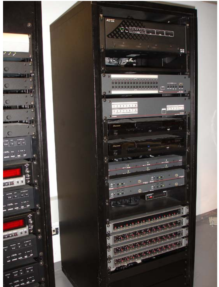
Equipment Rack with Extron Matrix Switchers and Twisted Pair Extenders
