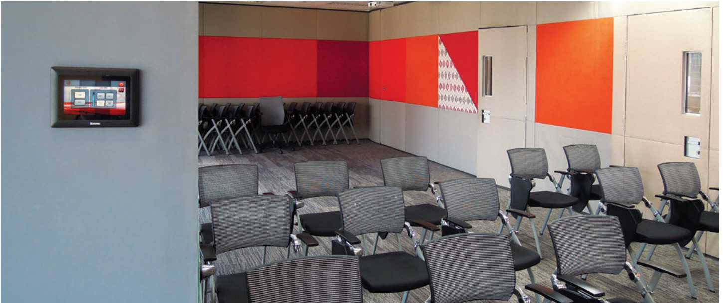
Each divisible training room provides a Pro Series TouchLink touchpanel mounted to a fixed wall, optimizing room configuration flexibility. Photograph courtesy of PT AIA Financial (AIA).
